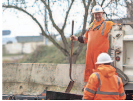
City workers place concrete barriers under the Marion Street Bridge in Salem on Wednesday.
