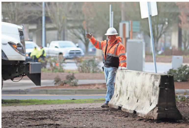
City workers place barriers under the Marion Street Bridge. This comes a day after police and social service providers cleared a homeless camp of an estimated 15 to 30 people from beneath the bridge.
