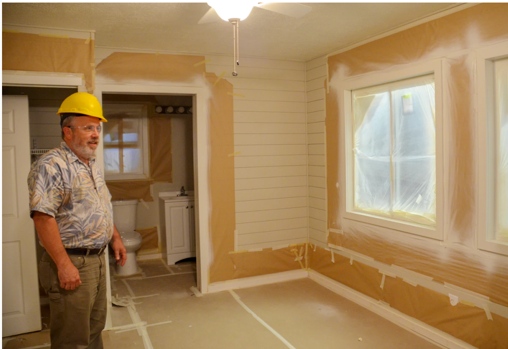
Ron Hays, CEO of United Way of the Mid-Willamette Valley, visits a tiny home under construction at 20 Twenty in Salem (Rachel Alexander/Salem Reporter)
