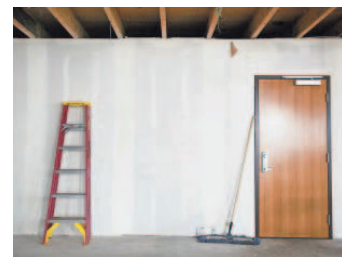
Part of the new ARCHES Project facility on Commercial Street was still under construction on Tuesday. This space will become part of the kitchen and pantry. The door opens to the newly opened day center.
